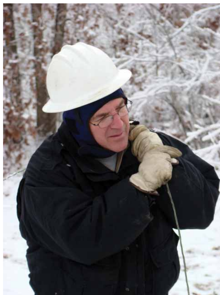
MIKE TRUETT, above left, works from a bucket truck as ice coats the Jackson Energy pick-up truck parked nearby. Truett was making repairs in Jackson County. Eddy Judd, above, pulls electric line across a field and up to a broken pole.
